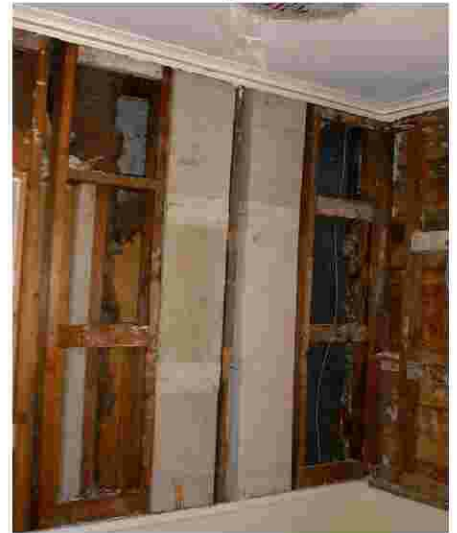
Demolition of the walls in this living room revealed Asbestos covered duct, running behind the old wall from the basement up to the second floor.
